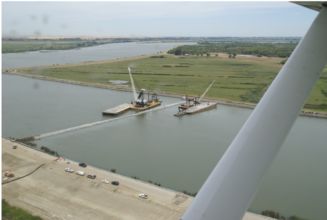
Photo 1: Partially constructed barrier and eastern edge of Jersey Island staging area during EDB installation (May 28 2015).
